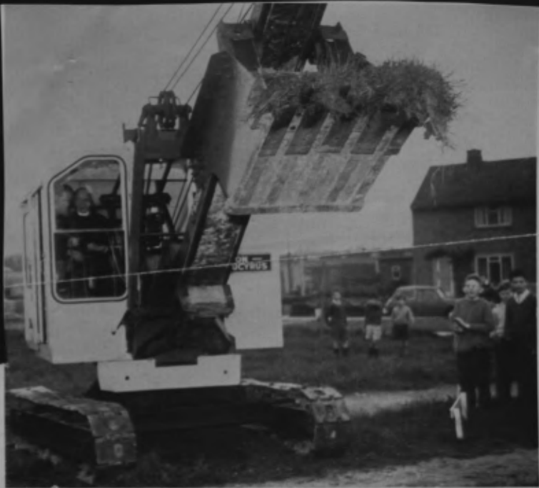
With Canon Cook at the controls, a 10-RB skimmer makes the first dig for the foundations of the new church on the Ermine Estate, Lincoln
